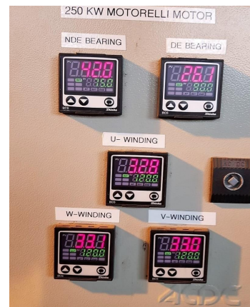
Example PT100 relay panel
